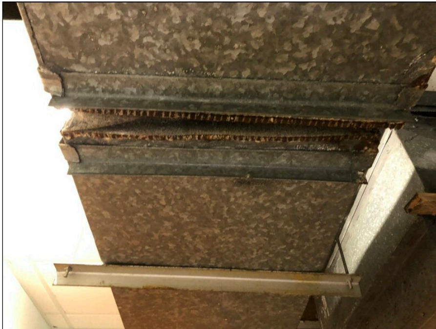
8 - View of HVAC Vibration Dampener
