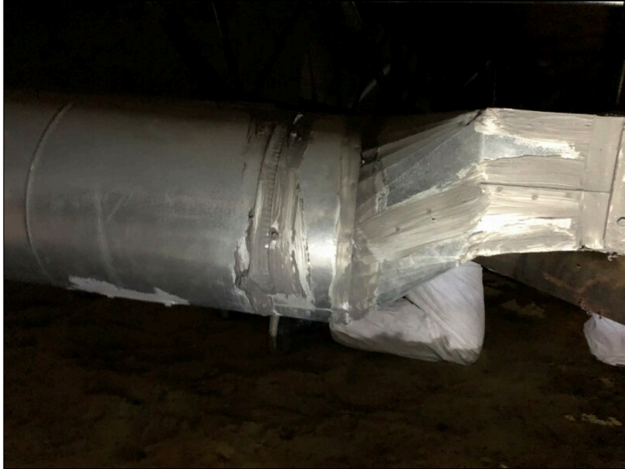
7 - View of Gray Mastic on Duct Work
