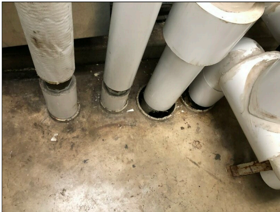
4 - View of TSI and Pipe Elbows
