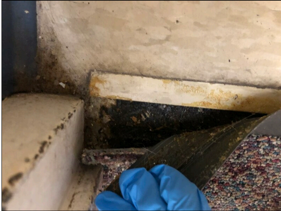
3 - View of Black Mastic Under Carpet
