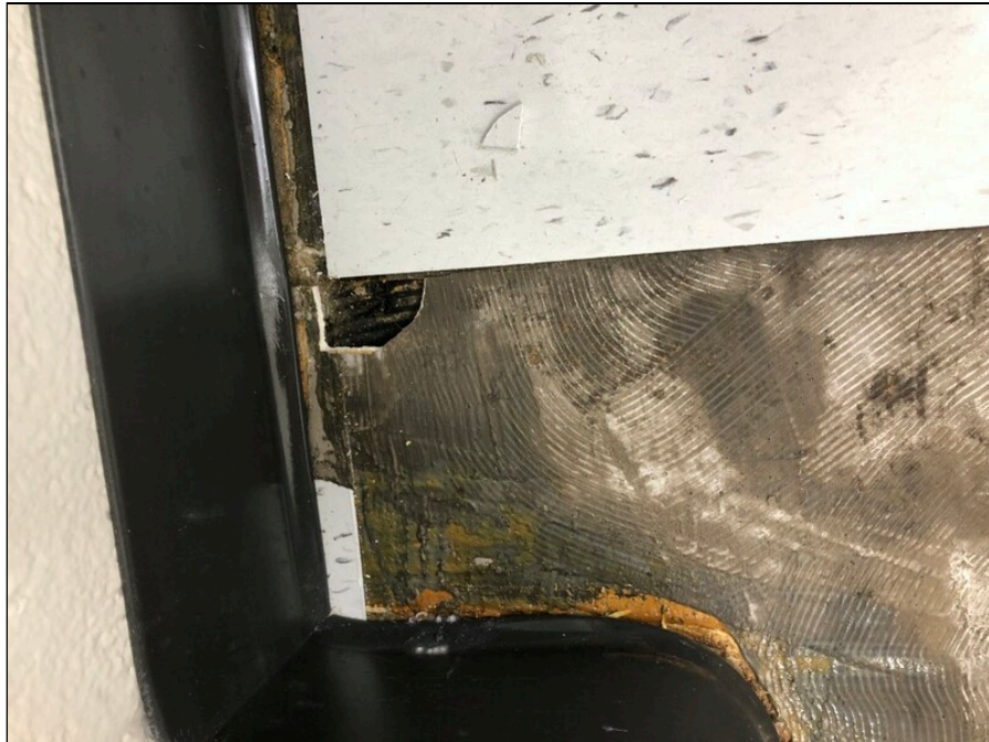
9 - View of Layered Tiles over Assumed ACM Black Mastic
