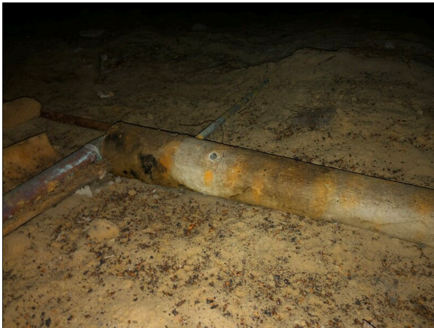
6 - View of Degraded TSI
