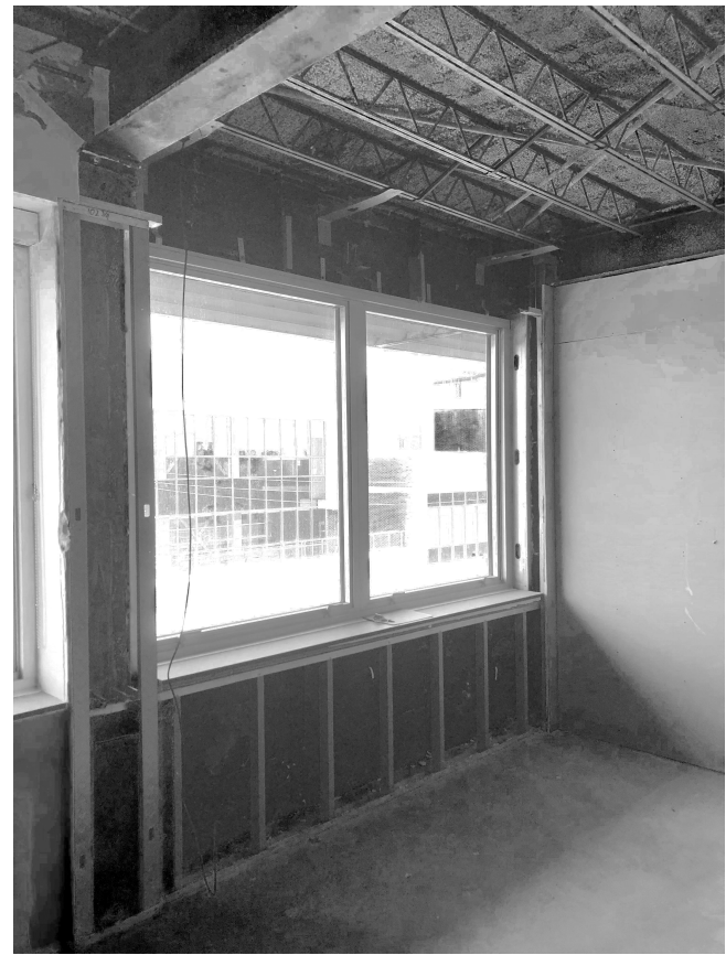
Condition at Key Note 2
